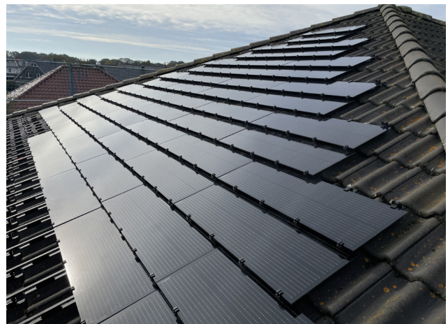
The SOLo system on the roof
